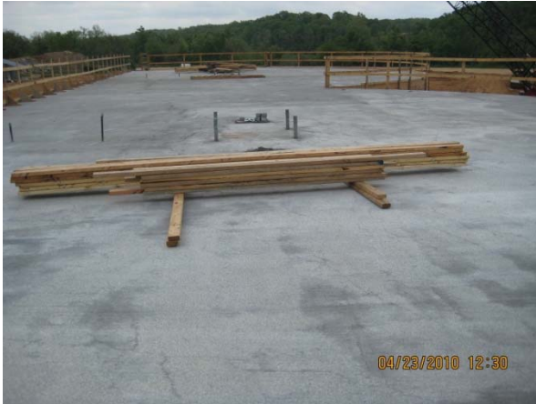
South decks of Process Trains 41 & 42
