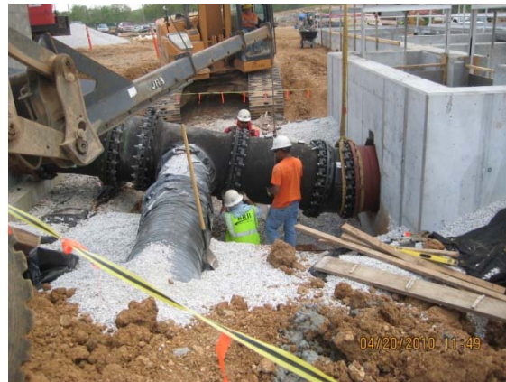
36" piping between Grit Chamber and Process Train
